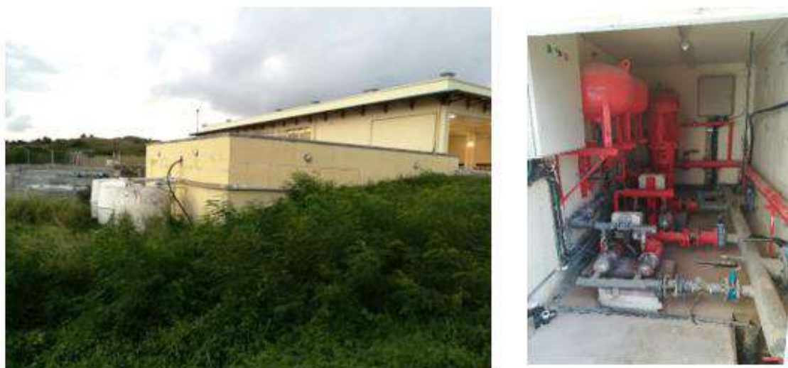
Figure 77: Water storage and distribution facilities at the airport passenger terminal building
