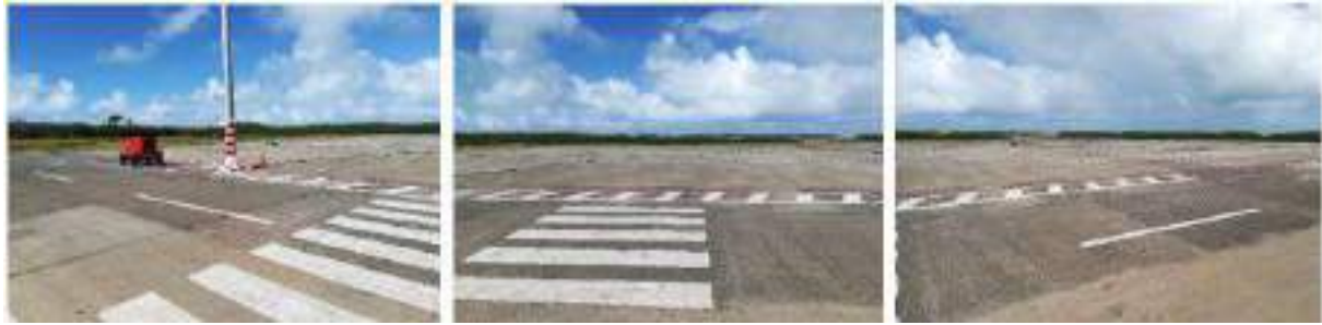
Figure 64: View of the existing drains observed around the apron in front of the passenger terminal building
