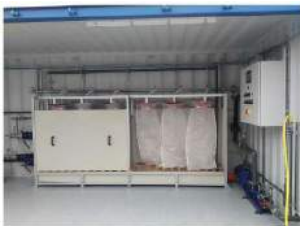
Figure 23: Example of the filtration bag technology proposed for the sludge treatment on site
